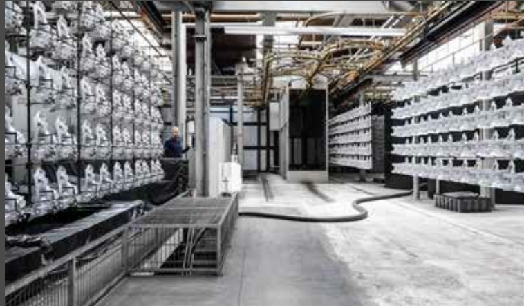
E-coating line for aluminium components (max. 7,000 x 2,400 x 500 mm)
